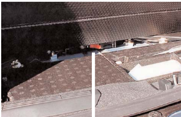
Capacitor Module Main Switch
